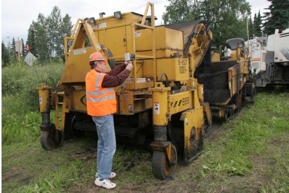
Figure 5: Construction paver, CAT AT-1055. Mike Ronchetti is attaching an RF reader. Photo by Janet Burton, University of Alaska.
