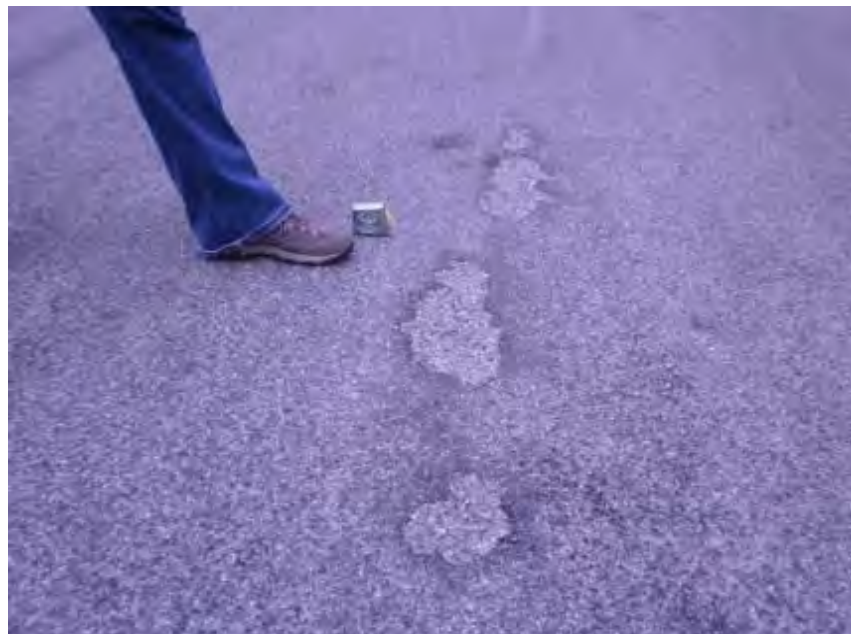
Figure 4-6. Bellevue Ave, Anchorage, double chip seal applied in 2010, bleeding, snowplow damage, and surface wear through the chip seal, photo taken in 2011
