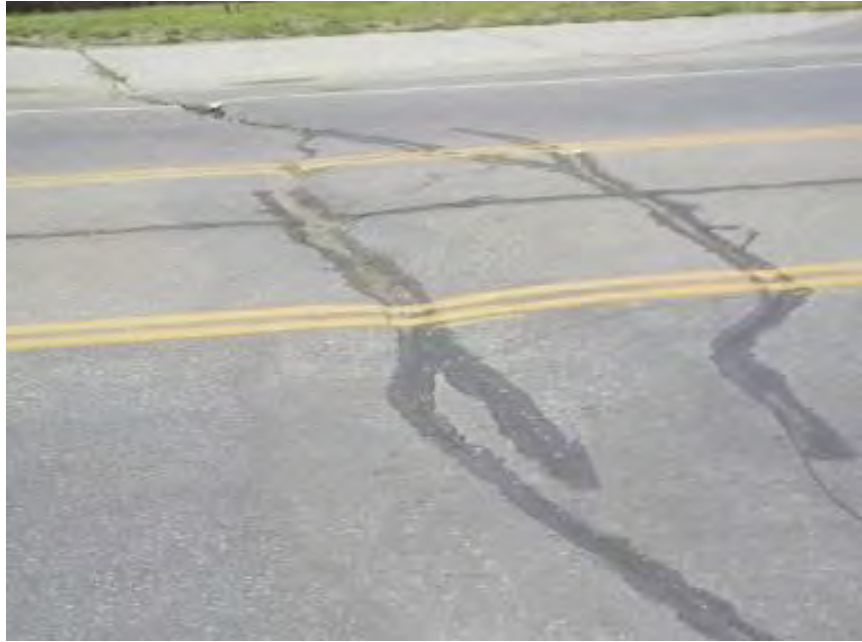
Figure 4-31. South Cushman St, Fairbanks, crack seal in 2011
