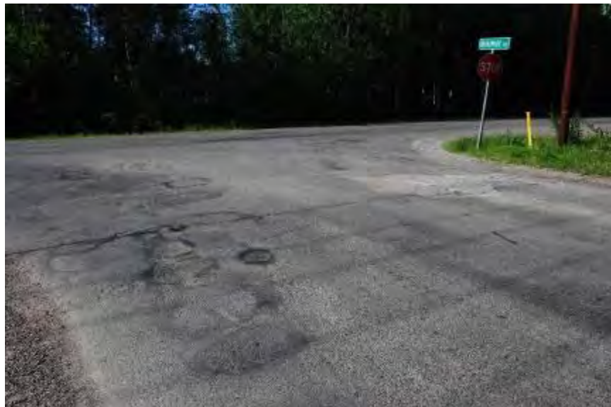
Figure 4-23. Broadmoor Ave between Dale Rd and Beechcraft Ave, Fairbanks, single C chip AST (before application), thermal cracking, patches, potholes, and raveling, photo taken in 2011
