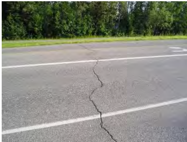
Figure 4-12. Farmers Loop Rd between Fairweather Rd and Summit Dr, Fairbanks, chip seal applied in 2008, photo taken in 2011
