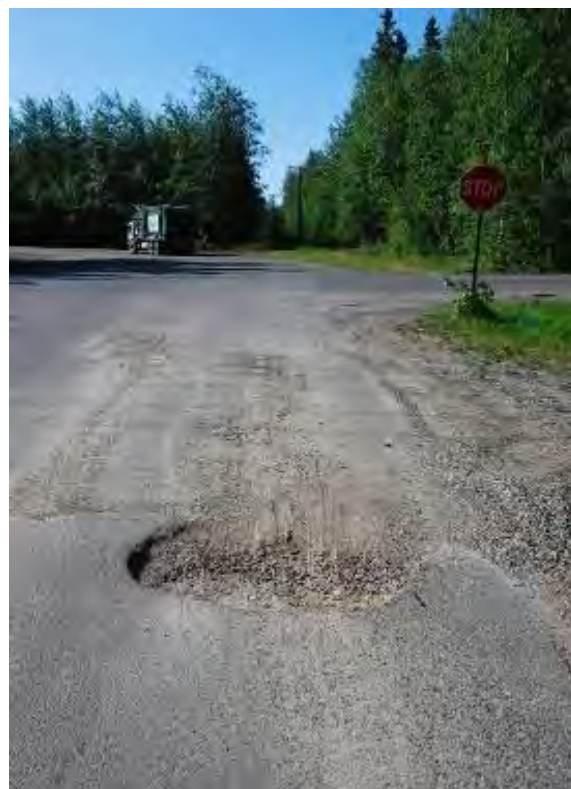
Figure 4-25. Western Ave between Dale Rd and Beechcraft Ave, Fairbanks, single C chip AST (before application), thermal cracking, potholes, and degrading permafrost, photo taken in 2011
