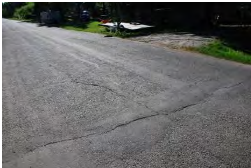
Figure 4-36. Teal Ave between Fairbanks St and Ramola St, Fairbanks, single C chip AST applied in 2011, thermal cracking, patches, potholes, and degrading permafrost, photo taken in 2011
