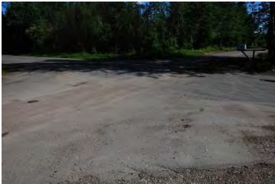
Figure 4-19. Mack Blvd between Morgan Way and Old Pioneer Way, Fairbanks, single C chip AST (before application), thermal cracking, patches, potholes, and degrading permafrost, photo taken in 2011
