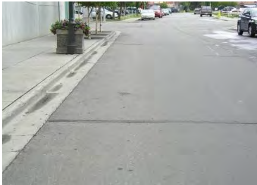
Figure 4-34. 3rd Ave, Fairbanks, crack seal, thermal cracking in 2011
