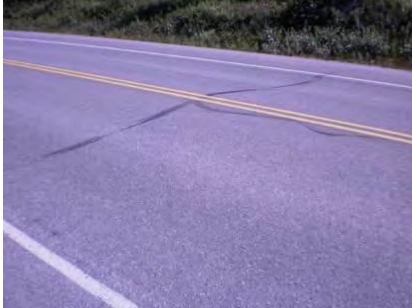
Figure 4-27. Abbott Rd, Anchorage, crack seal, thermal crack and frost damage, photo taken in 2011
