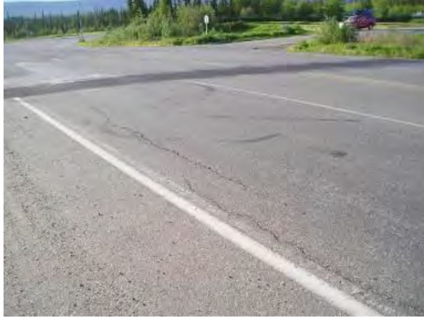
Figure 4-95. Farmers Loop Rd. between Steese Highway and Farmers Loop Ext, Fairbanks, chip seal applied in 2008, photo taken in 2011
