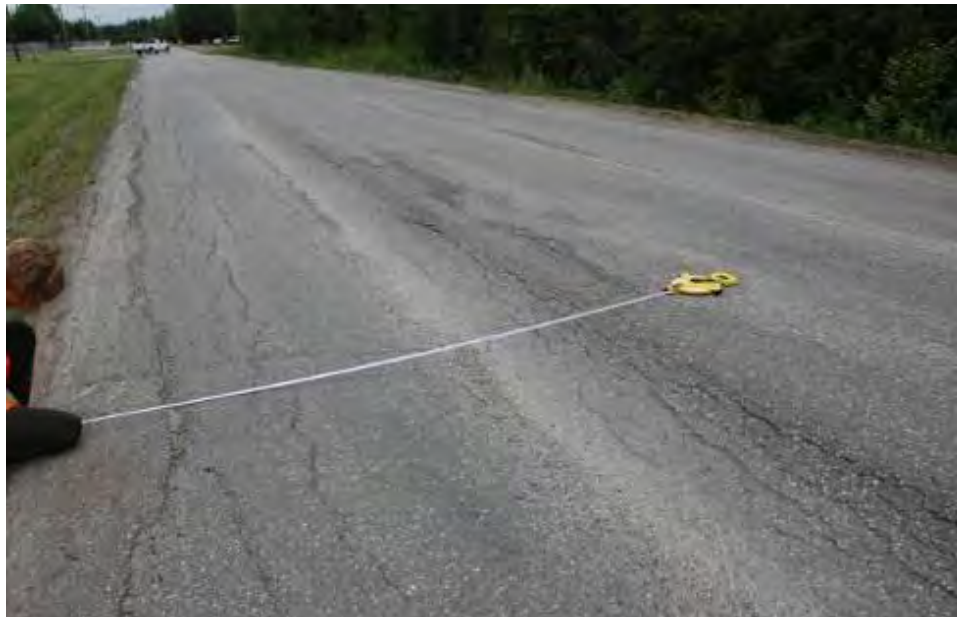
Figure 4-14. H&H Rd, North Pole. Rutting, transverse cracking, wheel path cracking, and permafrost degradation just prior to thin HMA overlay placed in 2011
