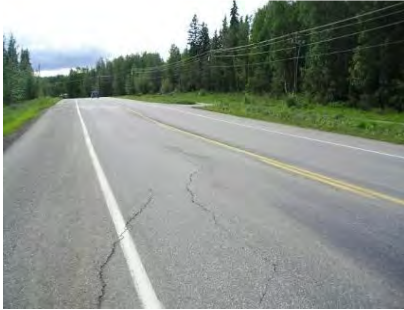
Figure 4-13. Farmers Loop Rd between Viewpoint and Scenic Hts, Fairbanks, double chip seal applied in 2008, thermal cracking, patches, degrading permafrost, photo taken in 2011
