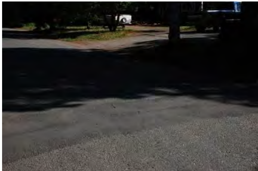
Figure 4-18. Halvorson Rd between Goldizen Ave and Widener Ln, Fairbanks, single C chip AST applied in 2011, thermal cracking, patches, and degrading permafrost, photo taken in 2011
