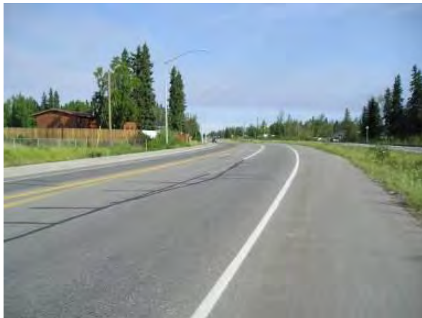
Figure 4-30. Trainor Gate Rd, Fairbanks, crack seal in 2011
