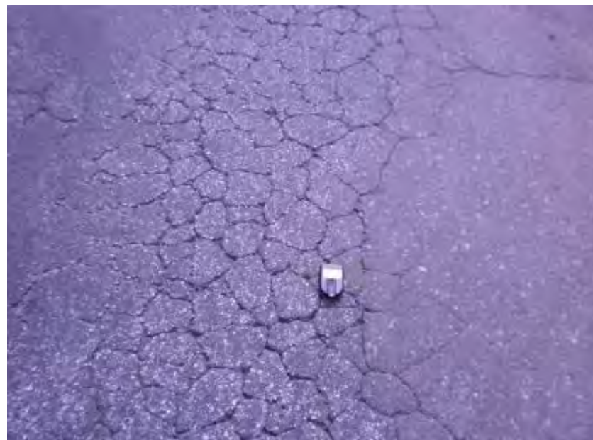
Figure 4-8. Pioneer Ave, Anchorage, double chip seal applied in 2003, fatigue cracking in wheel path, photo taken in 2011
