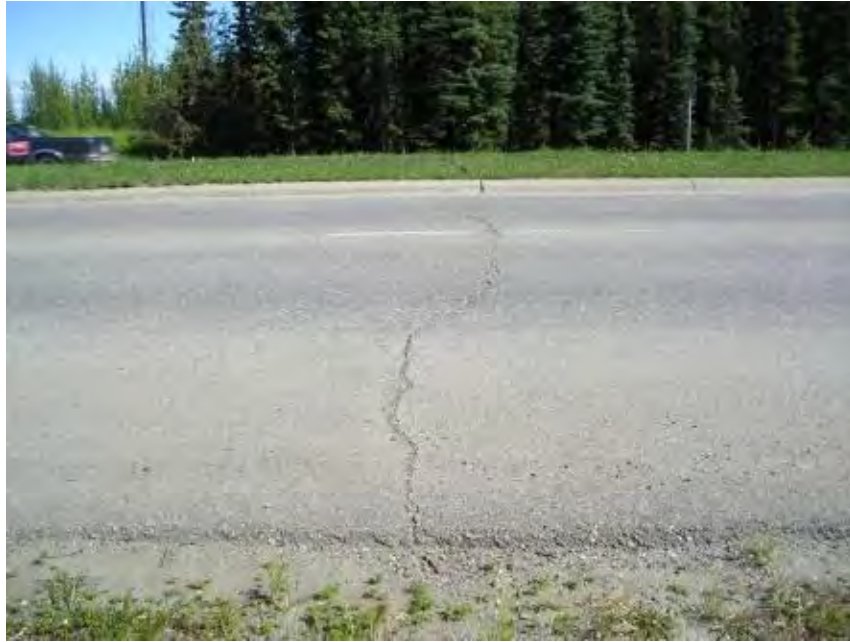
Figure 4-17. Farmers Loop Rd between Taku and College, Fairbanks, double chip seal applied in 2008, thermal cracking and center joint cracks, photo taken in 2011
