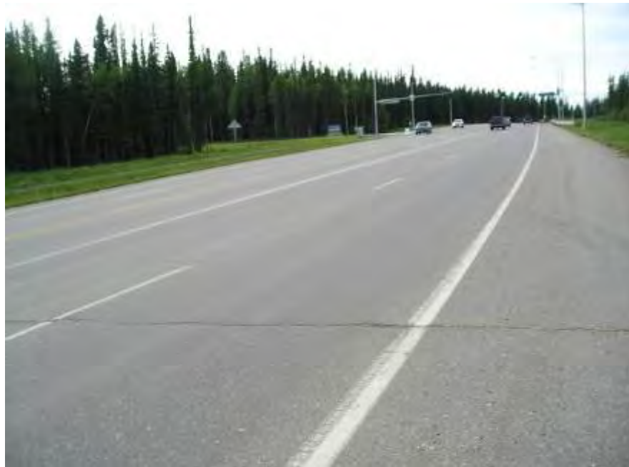
Figure 4-16. Farmers Loop Rd between Tanana and Taku, Fairbanks, double chip seal applied in 2008, thermal cracking and center joint cracks, photo taken in 2011
