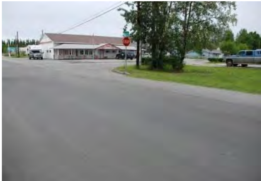
Figure 4-10. Snowman Lane, North Pole. Transverse cracking just prior to thin HMA overlay, 2011
