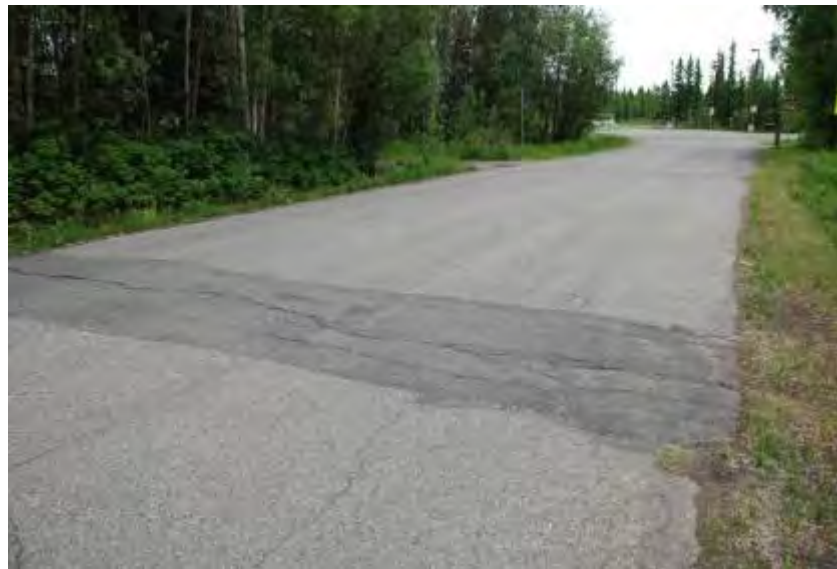
Figure 4-12. Davis Blvd, North Pole. Transverse cracking and permafrost degradation, 2011
