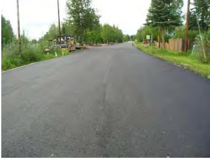
Figure 4-11. Snowman Lane, North Pole. Just after thin HMA overlay placed in 2011
