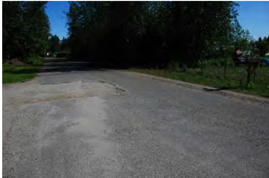
Figure 4-21. Old Pioneer Way between Luke St and Mack Blvd, Fairbanks, single C chip AST (before application), thermal cracking, patches, large pothole, and degrading permafrost, photo taken in 2011
