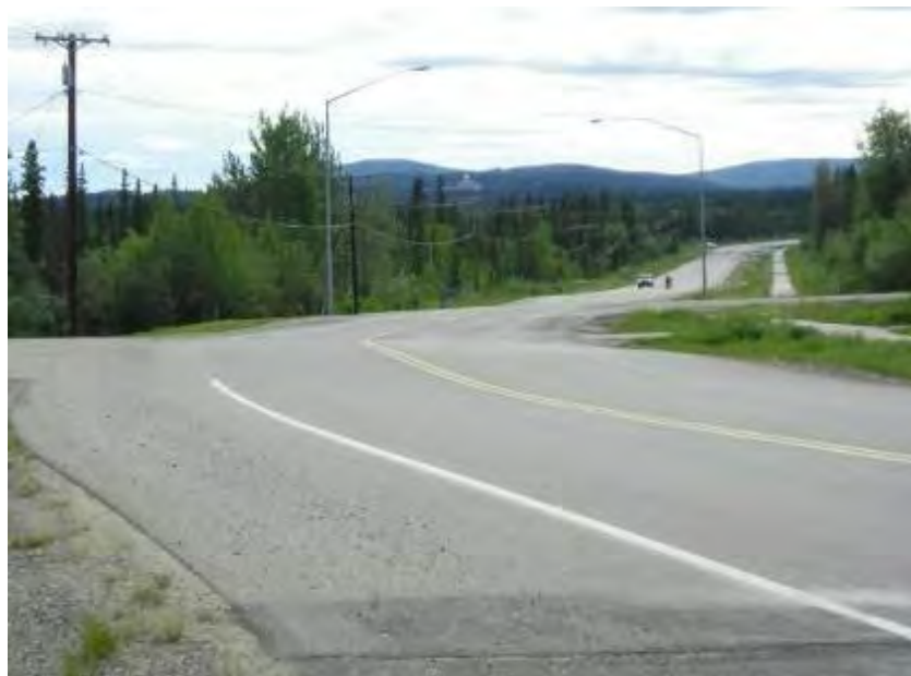
Figure 4-30. Farmers Loop Rd between Grenac and Viewpoint, Fairbanks, double chip seal applied in 2008, thermal cracking, patches, permafrost, photo taken in 2011
