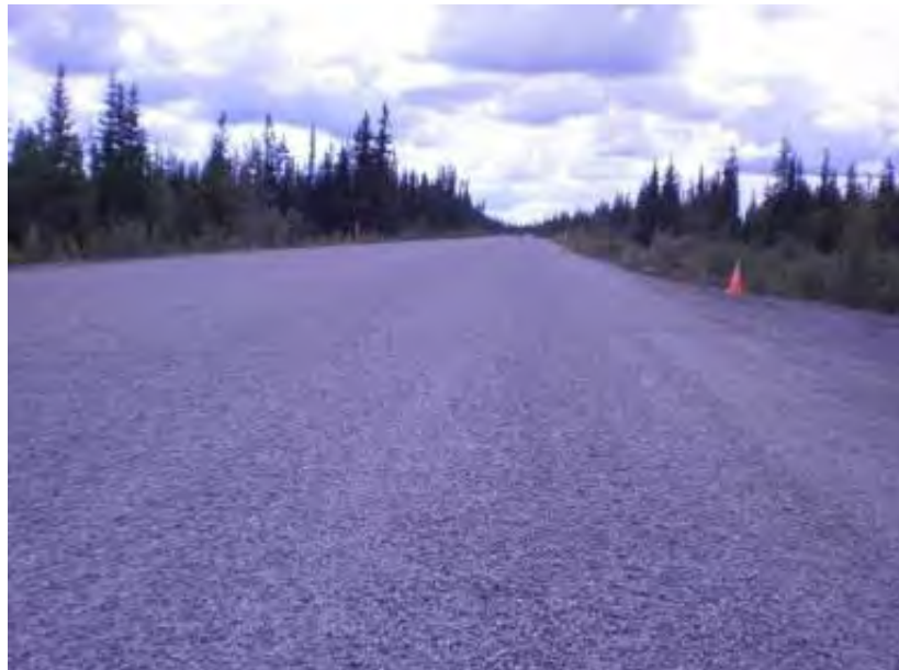
Figure 4-26. Tok Cutoff, Gokana, Double chip seal over cold in place recycling, photo taken in 2011
