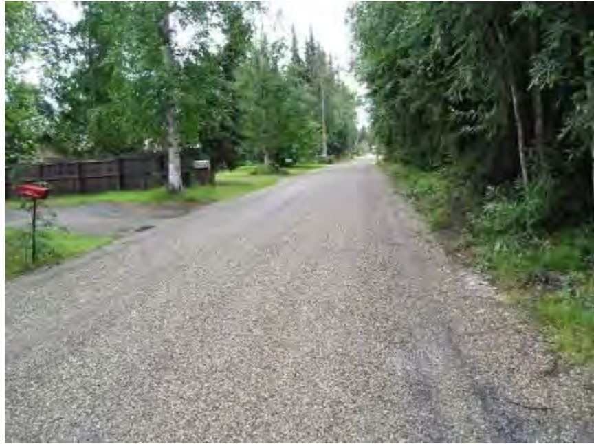
Figure 4-39. Halvorson Rd between Goldizen Ave and Widener Ln, Fairbanks, single C chip AST applied in 2011, post application, photo taken in 2011
