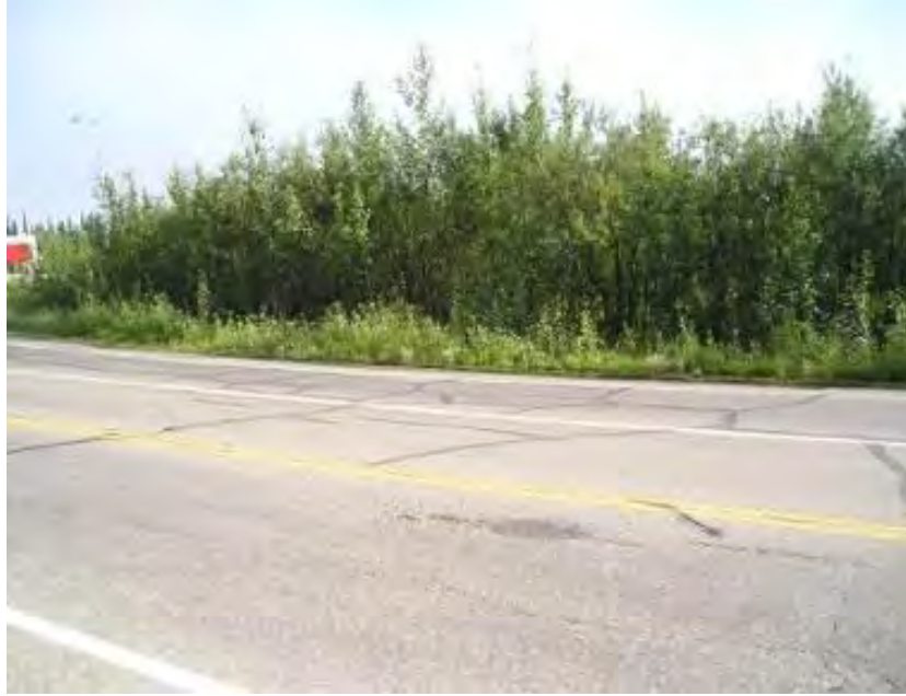
Figure 4-29. Wembley Ave, Fairbanks, crack seal in 2011
