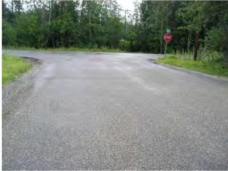
Figure 4-24. Broadmoor Ave between Dale Rd and Beechcraft Ave, Fairbanks, single C chip AST applied in 2011, post application, photo taken in 2011
