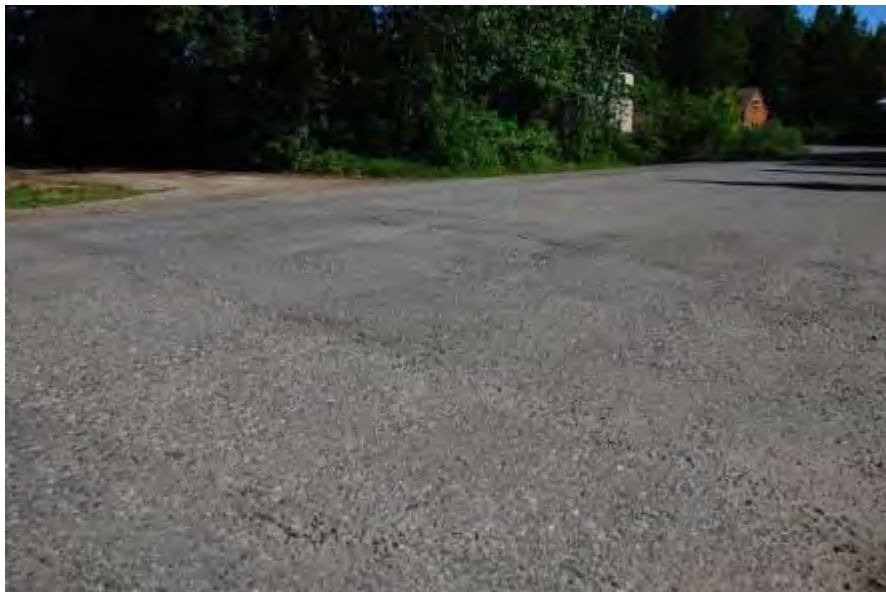
Figure 4-44. Totem Dr between Morgan Way and Luke St, Fairbanks, single C chip AST (before application), thermal cracking, patches, raveling, and degrading permafrost, photo taken in 2011
