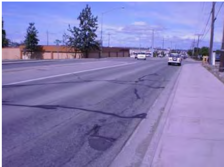
Figure 4-28. Old Seward Highway, Anchorage, crack seal, thermal and frost cracking, photo taken in 2011
