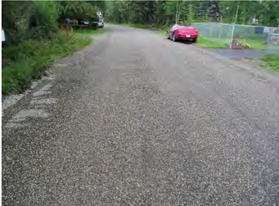
Figure 4-22. Totem Dr between Morgan Way and Luke St, Fairbanks, single C chip AST applied in 2011, post application, photo taken in 2011
