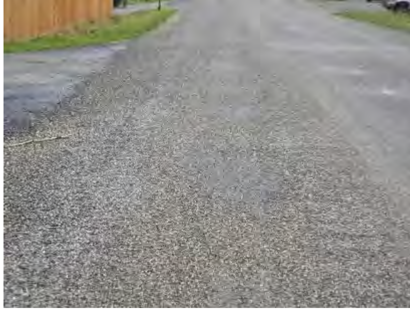
Figure 4-49. Western Ave between Dale Rd and Beechcraft Ave, Fairbanks, single C chip AST applied in 2011, post application, photo taken in 2011
