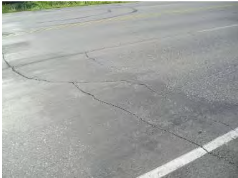
Figure 4-10. Farmers Loop Rd between Spur Rd and McGrath Rd, Fairbanks, chip seal applied in 2008, photo taken in 2011
