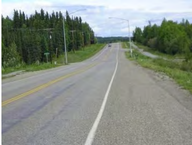
Figure 4-29. Farmers Loop Rd between Summit Rd and Grenac, Fairbanks, double chip seal applied in 2008, potholes and permafrost damage, photo taken in 2011
