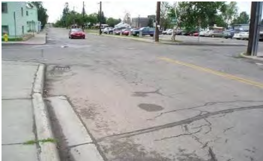
Figure 4-32. Lacey St, Fairbanks, crack seal, thermal cracking, alligator cracking, and degrading permafrost, 2011
