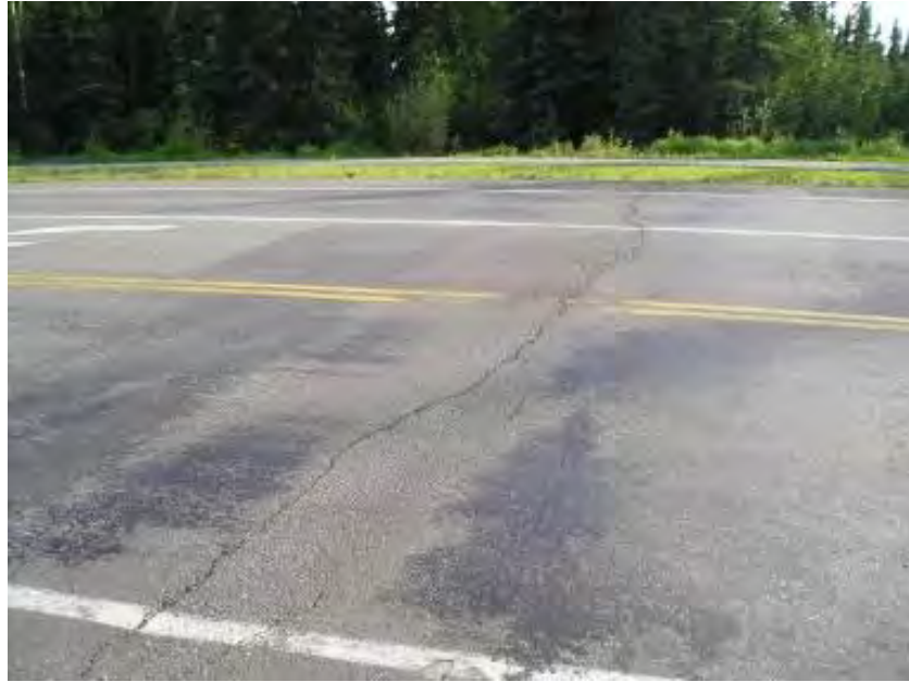
Figure 4-11. Farmers Loop Rd between McGrath Rd and Fairweather Rd, Fairbanks, chip seal applied in 2008, photo taken in 2011
