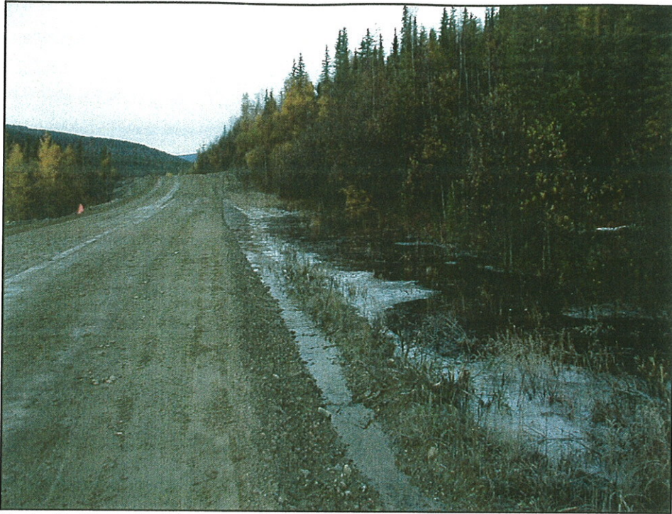
Photo 9. View looking west from MP 86.9 Taylor Highway. Typical drainage along the Wade Creek Section of road. (9/12/02).
