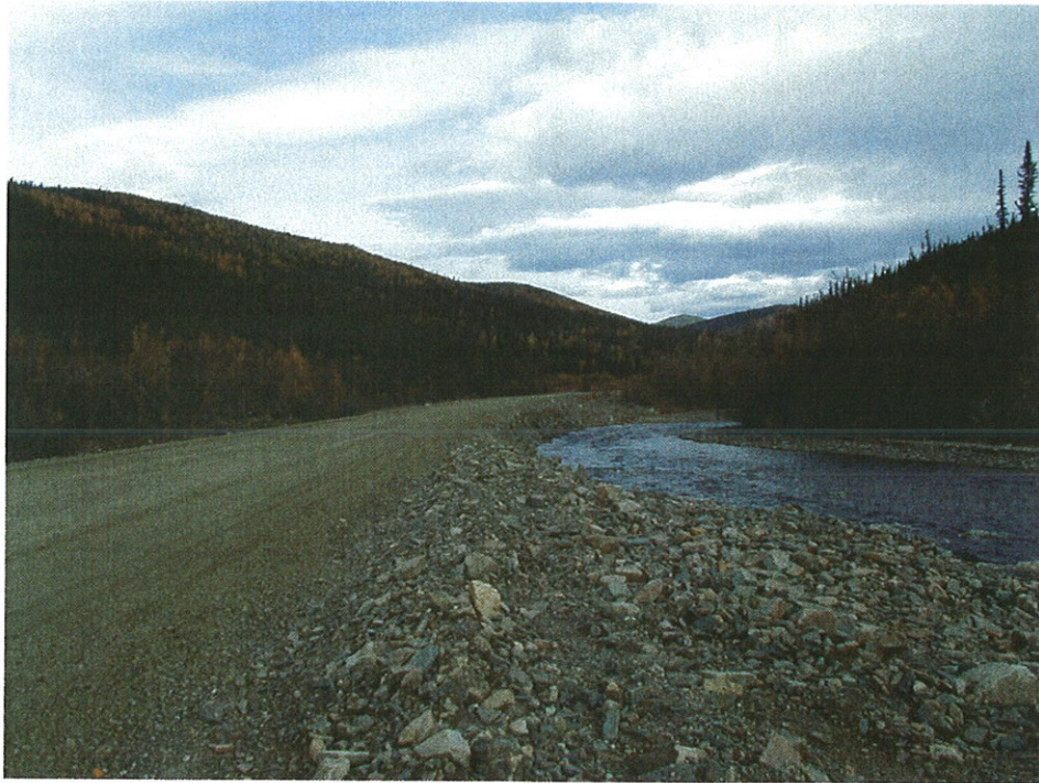
Photo 6. Erosion of the Taylor Highway by Wade Creek. (9/12/02)
