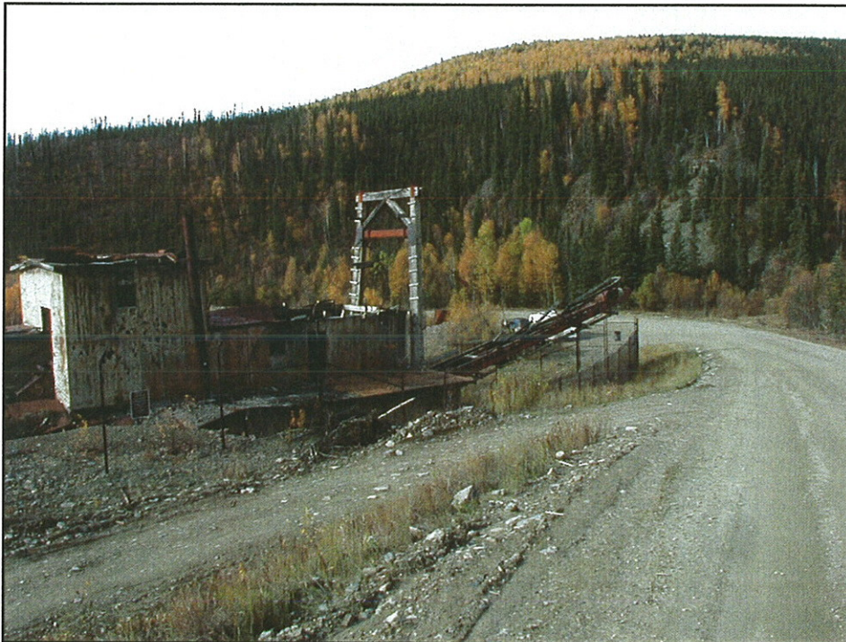
Photo 4. Jack Wade Dredge, MP 86 Taylor Highway. Dredge is proposed to be dismantled by BLM, date for dismantlement has not been set. Road will be widened away from dredge. (9/12/02).
