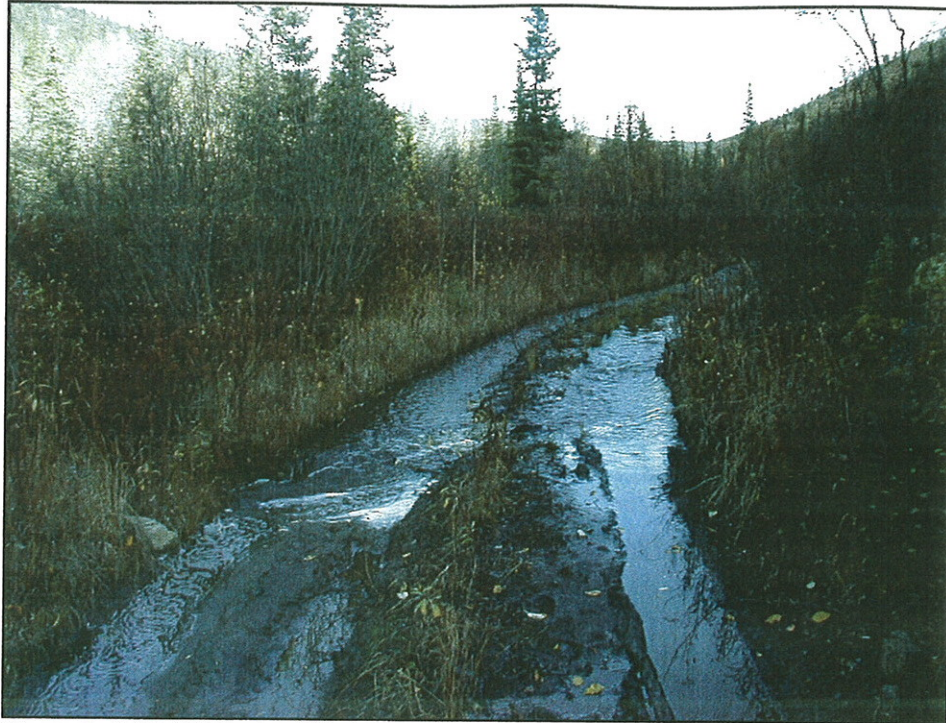
Photo 7. MP 90 Taylor Highway. Typical drainage problem along a side road of the highway near Wade Creek. (9/11/02).
