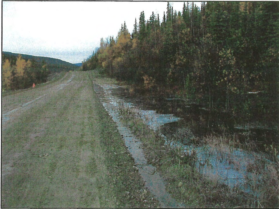
Photo 3. View looking west from MP 86.9 Taylor Highway. Typical drainage along the Wade Creek Section of road. (9/12/02).
